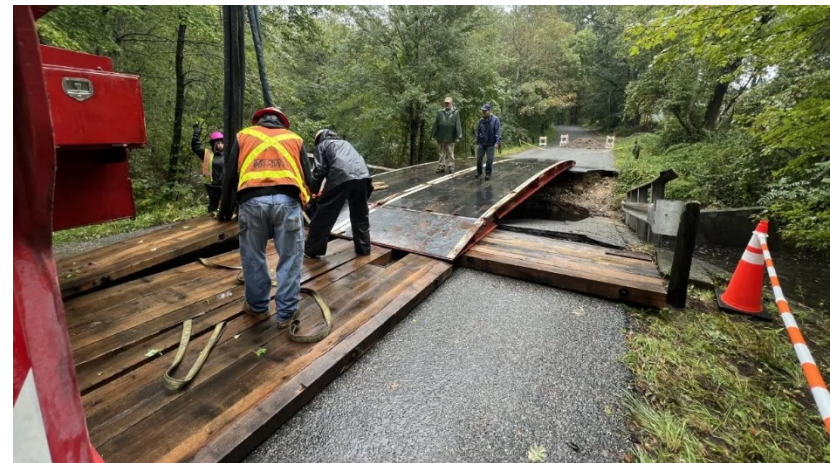
Temporary ramp installed over washed out bridge in Scotland, 2023. Image taken from NBC CT.
